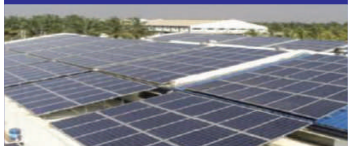
600 KWp-at Eppineger Coimbatore 180
